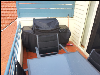
Tiled Balcony is leaking into garage below
