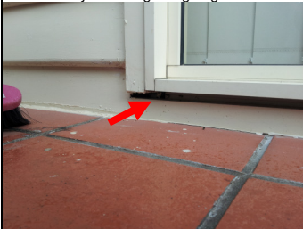
No evidence of flashing (upstand) at door sill
