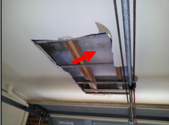
Substrate is cement sheet and should be able to be retained for re-use.
