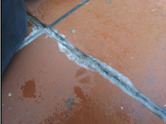
Water is entering substrate via grout and is pooling between membrane and tile as evidenced by water deposited minerals in the grout.
